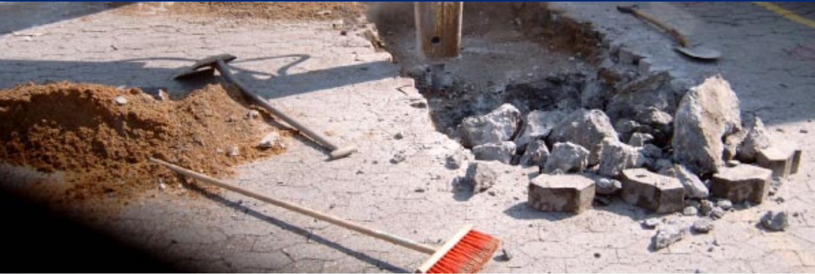
Portable Falling Weight Deflectometer (LWD) is applied for measurement on many different pavement surfaces.
